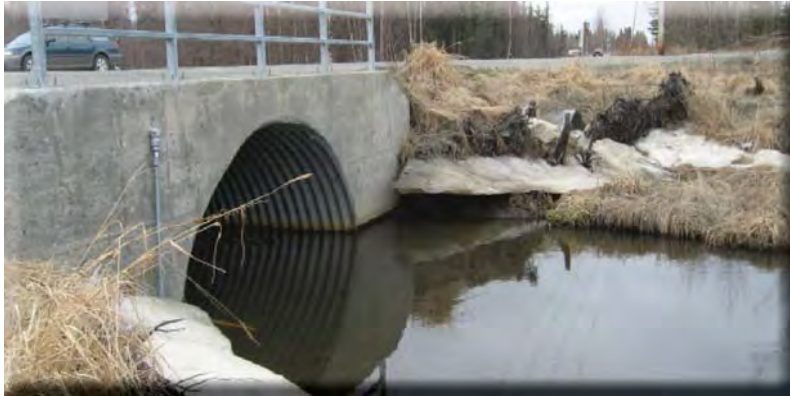
Storm drain system
